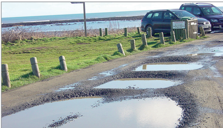
Boulmer Beach Car Park. This was the state of the car park a few years ago. It costs money to maintain a facility of this sort which is used by people from all over the county.
